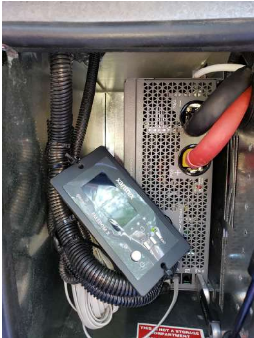
2021 Unity Bluetooth Remote Cable Tied to 120vAC cables in the Inverter Bay
